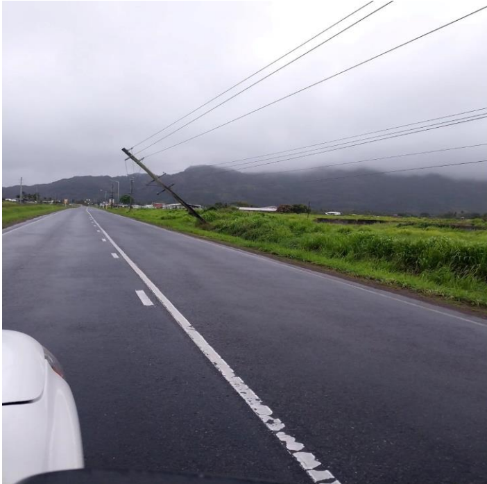
Figure 6a: Isolated disruption in electricity supply due to damaged power lines (Sabeto, Highway)
